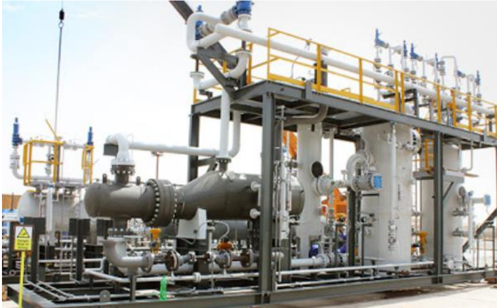
Figure 5.9 Typical Gas Enrichment (Amine) Plant in Biogas
