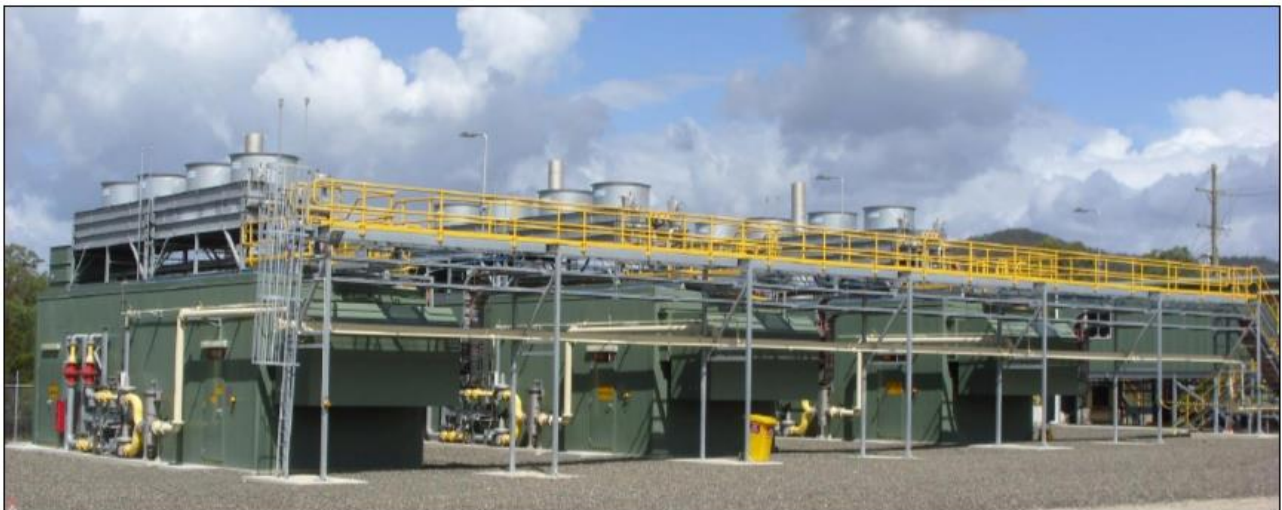
Figure 5.7 10 MW power station - 3 x 3.3 MW Gas Gensets
