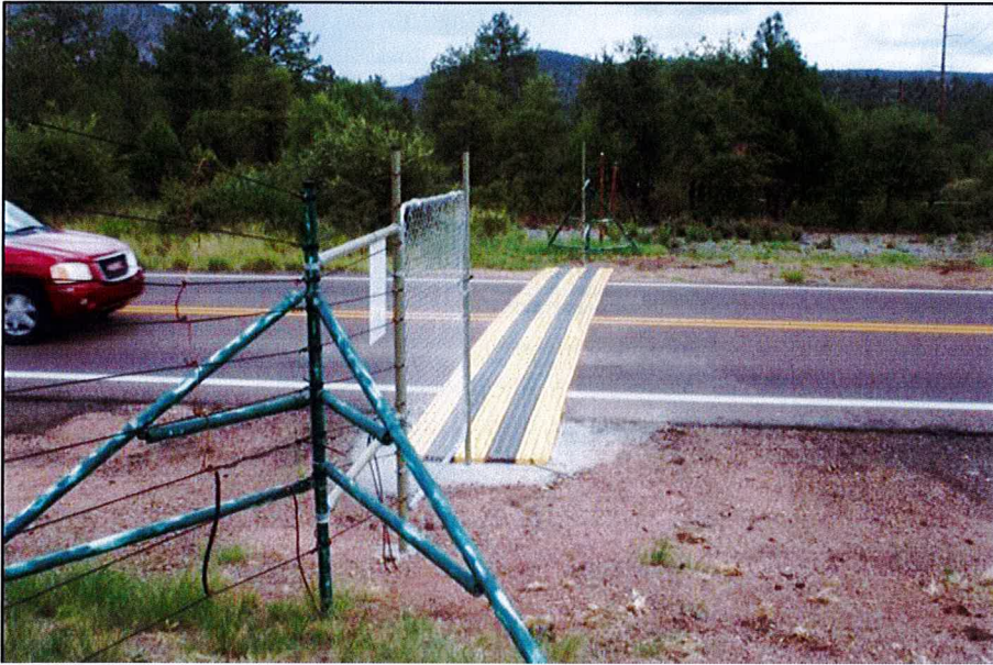
Figure 4.4 Electric mat deployed on an at-grade crossing in North America. (Gagnon et al. 2020)
