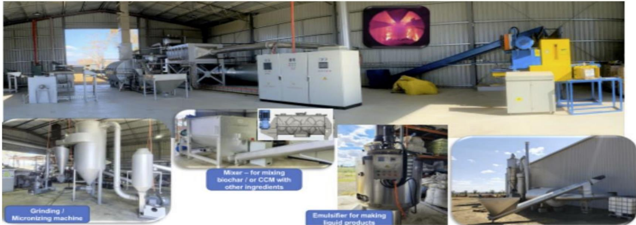
FIGURE 14 CARBON POWERED MINERAL COMPLEX FACTORY. LARGER SYSTEM SET UP ALSO NOW DEPLOYED.
