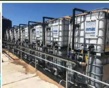
Stand alone filter system to filter metals from industrial sites. Photo by Ryan Holmann, Stormwater Biochar, filters by BioLogical Carbon
