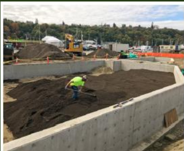
Stormwater vault. Photo by Sarah Burch
