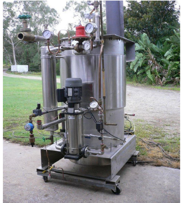
Figure 5. 0.5MW Pulse Combustion Steam Boiler
