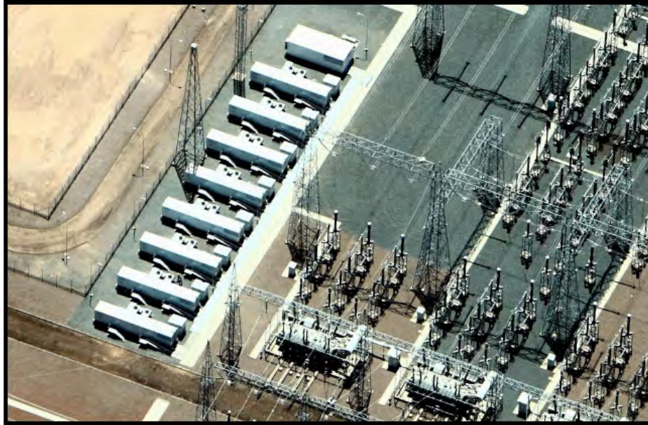
Figure 4-19 Commercial operation of a 12-MW frequency regulation and spinning reserve project at AES Gener's Los Andes substation in the Atacama Desert, Chile. The system uses A123 Systems' Li-ion Hybrid Ancillary Power Units (Hybrid-APUs™).
