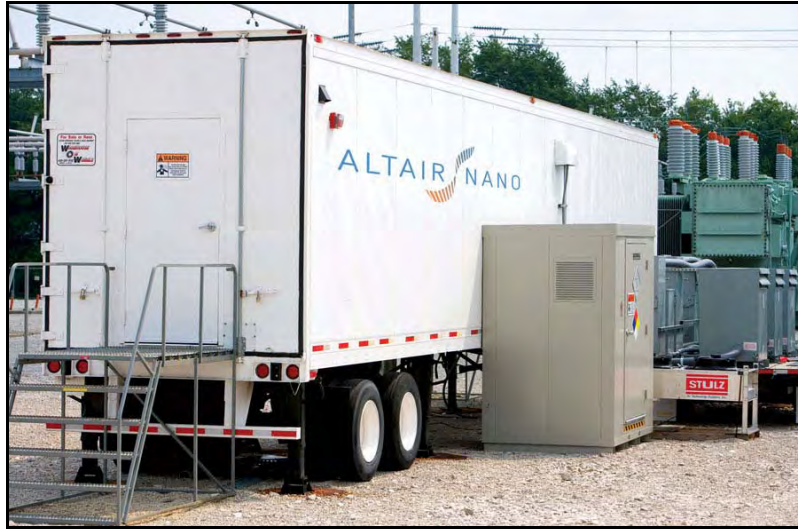
Figure 4-18 1-MW/250-kWh transportable Altairnano Li-ion energy storage system at PJM
