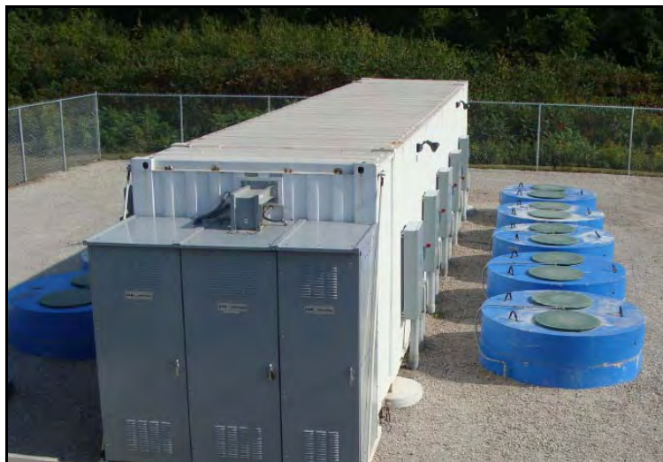
Figure 4-16 1-MW/15-min Beacon Power flywheel in an ISO ancillary service application
