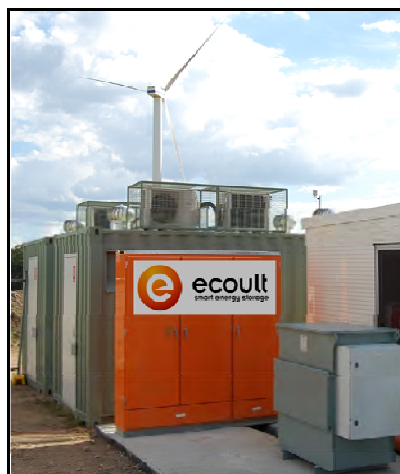
Figure 4-8 Phase 1 of Ecoult 1-MW/1-MWh UltraBattery system at Hampton Wind Smoothing Project in Australia (Source: Ecoult).
