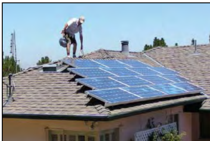
Figure 3-11 Residential Rooftop Photovoltaic Panels (Source: NREL)
