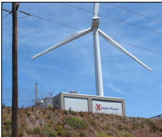
Figure 4-9 1.5-MW/1-MWh Advanced Lead Acid “Dry Cell” Systems by Xtreme Power being deployed in a wind farm application (Source: Xtreme Power).
