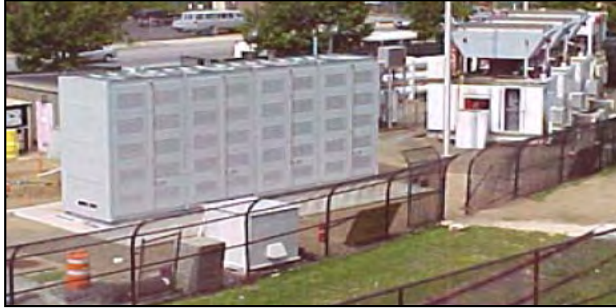
Figure 4-10 NYPA 1.2-MW/7.2-MWh Sodium-Sulfur Battery Facility
